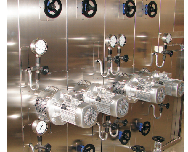
pict.1: thermoil pump system
